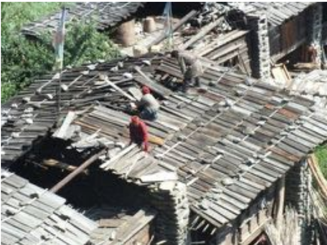
Photo 4: People rebuilding their house through the salvaged wood from their broken house, Gatlang, Rasuwa, 2015
