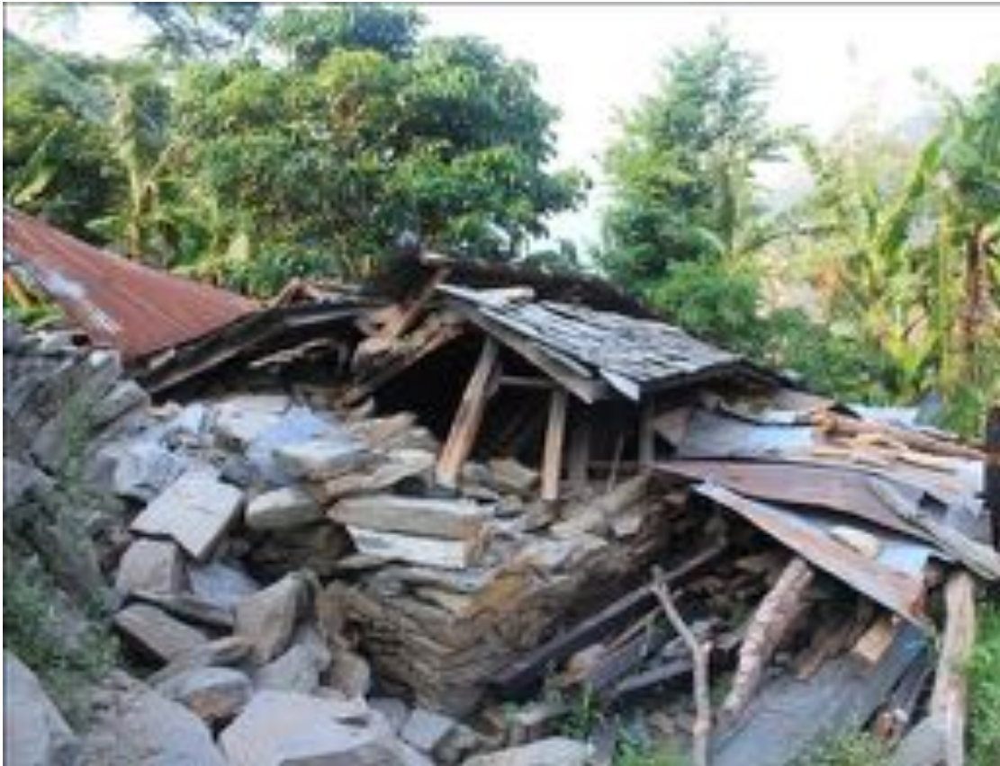
Photo 7: Destroyed conventional house in Jharlang, Dhading, 2015
